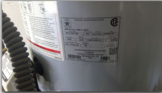
Water Heater Manufacturing Date
